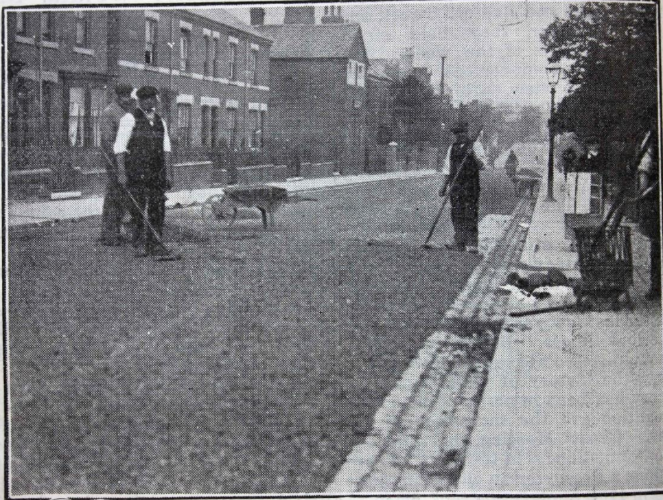
MOOR STREET, EARLSDON, SHOWING THE PATHS AND ROADWAY CONSTRUCTED OF MATERIAL FROM THE DESTRUCTOR WORKS.
